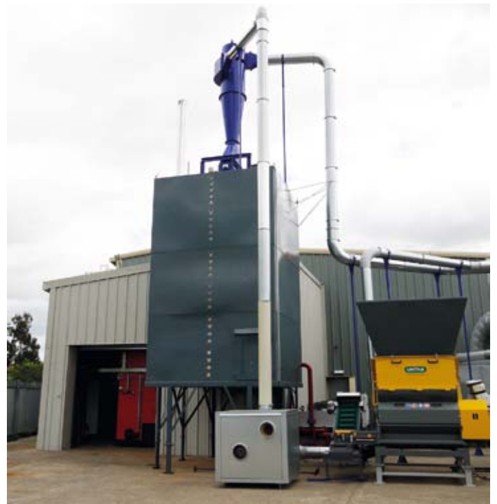
One of our new biomass boilers and hopper feed system.
